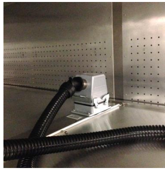
Figure 2-4 Canopy Wire Harness Connection
