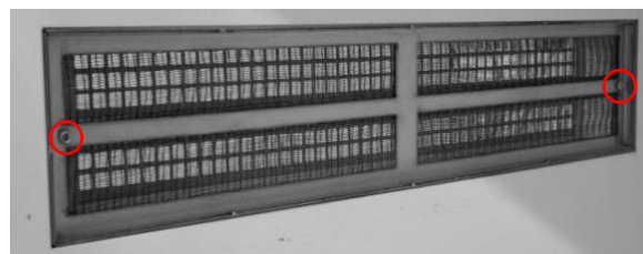
Figure 2-10 PC Canopy Air Inlet Filter Installed
