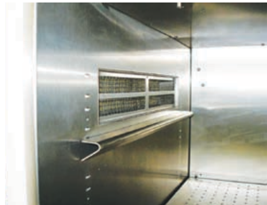
Figure 2.27: Air filter installed in its compartment. Again, notice the position of the lamp canopy support with respect to the filter.
