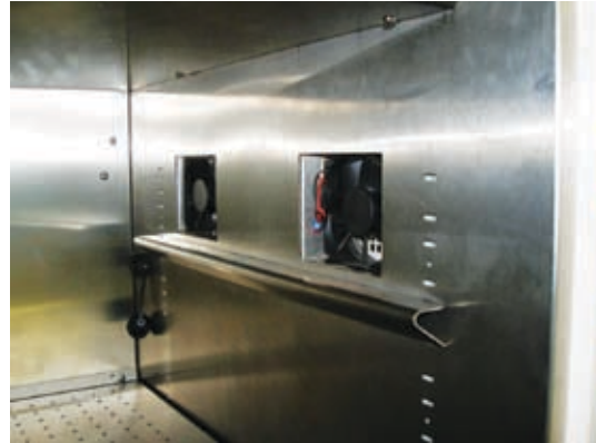
Figure 2.26: Fans installed and plugged in to their compartments. Notice the position of the lamp canopy support with respect to the fans.
