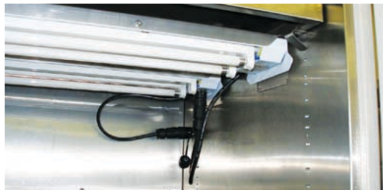
Figure 2.17: Lamp fixtures assembled and plugged.
