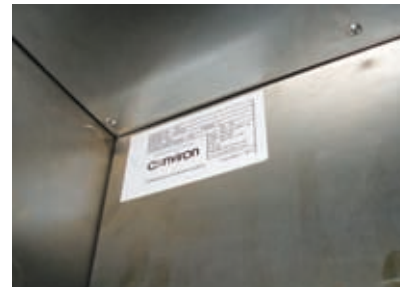
Figure 2.25: Shows in detail the back plenum installed above the fan housing.
