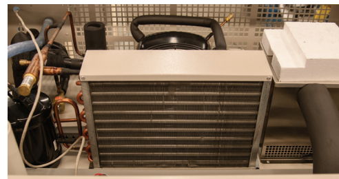
Figure 3.3: Air cooled condenser
